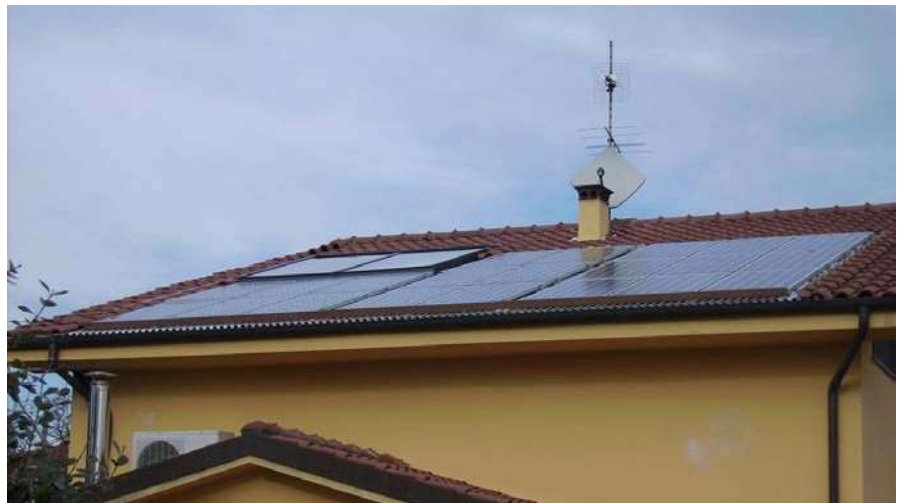
Image 99: Photograph of solar panels installed on the roof of a house in accordance with the technical building code.
