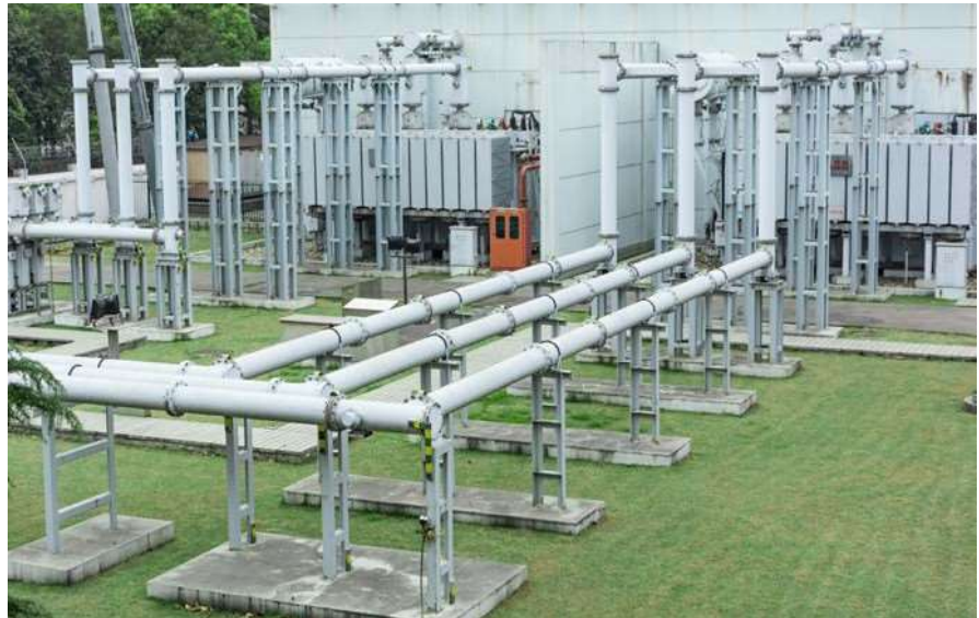
Figure 93: Photograph of a mini-hydropower plant.
